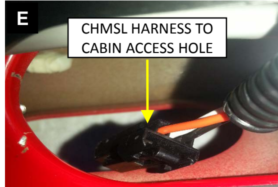
E CHMSL HARNESS TO CABIN ACCESS HOLE LED CHMSL – PREVENT LIGHT FLASH BACK INTO CABIN BY TAPING OVER ACCESS HOLE.
