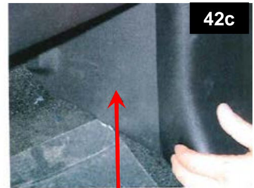
Fuse Box panel cover
